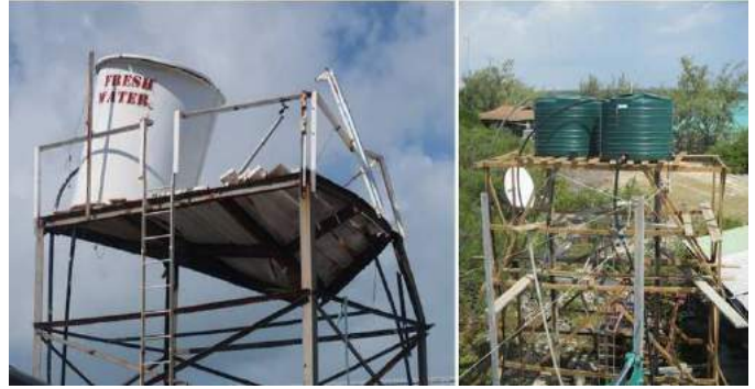
Collapsed water tower and the temporary wooden solution © SIF
